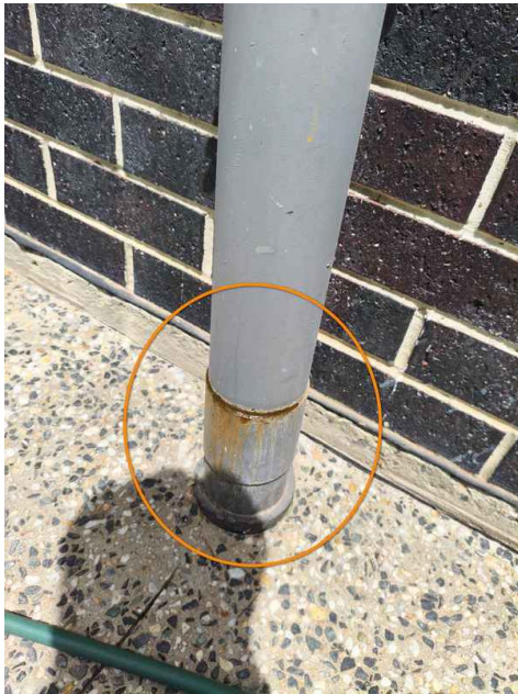
Connection failure observed as a result of movement in the concrete.
