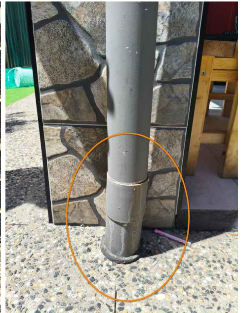
Connection failure observed as a result of movement in the concrete.
